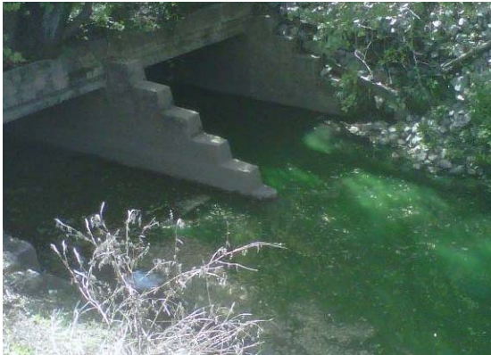
View of Illicit discharge to Jordan's Branch at Car Wash facility on West Broad St. April 2011.
